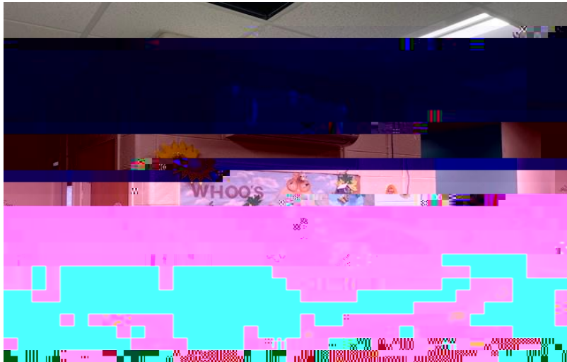
Great Hollow Middle School Unit Ventilation project- Ductwork installation on roof and Guidance Area Wall Pack installation
